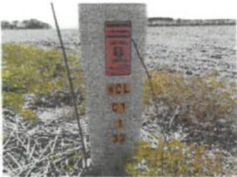
7. Telco at the road
