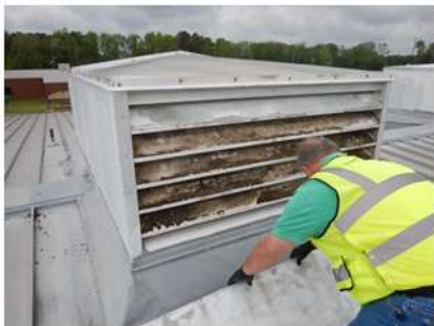
Fresh Air Intake Covered
