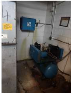
Pneumatic Controls Inop
