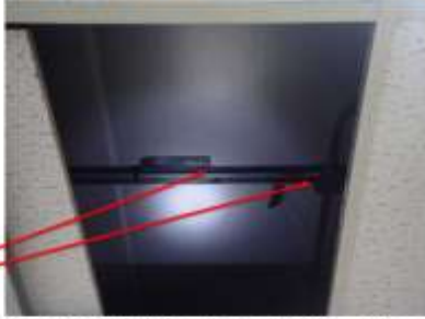
Liquid Water Dripping
